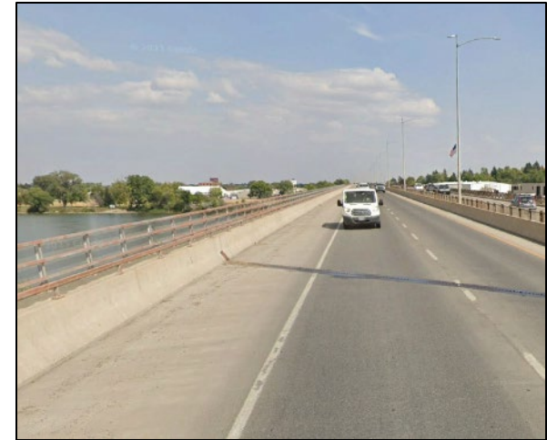
The westbound section of the Warden Bridge, on 10 th Avenue South spanning the Missouri River, is in poor condition while the eastbound section is in fair condition and has been noted as needing repair or replacement.
